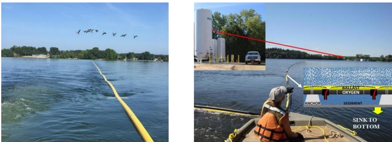
Figure 1. Left picture: Linear diffusers towed into place with weights installed (Vahanen; Jacobs, 2022). Right picture: Linear diffusers positioned over the design location and sinking gradually from shore as the ballast pipe filled with water. Note the liquid oxygen supply tank photo insert (Vahanen; Jacobs, 2022).
